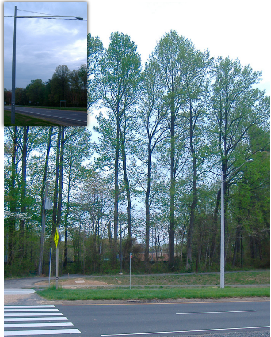
Street lights have been installed at the crosswalk
