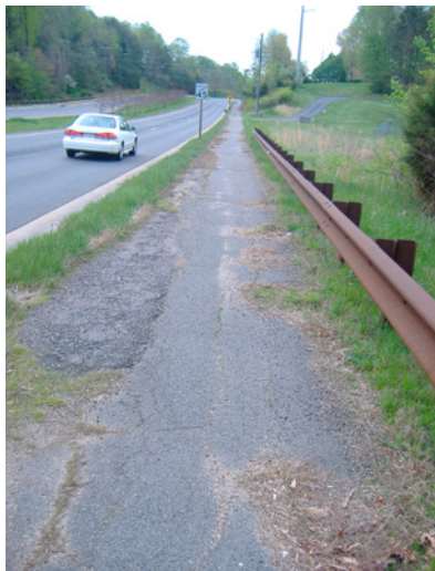
The existing trail is in disrepair
